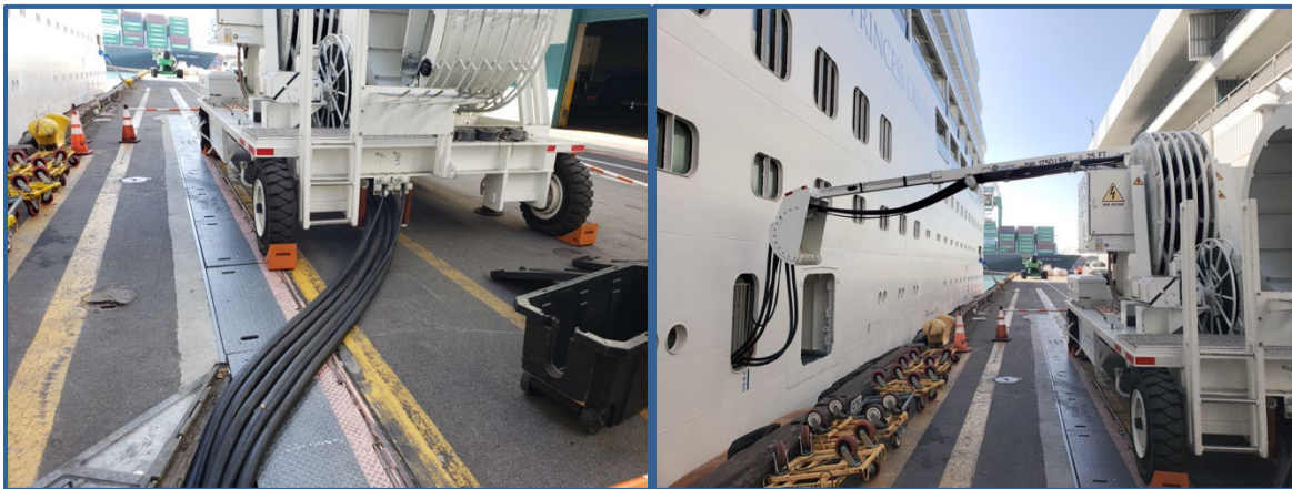
Figure 5: Mobile shore power cable reel (left) and vessel connection (right) at the Port of Los Angeles Source: Port of Los Angeles
