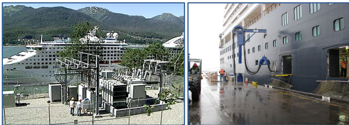
Figure 1: Electrical substation (left) and high voltage shore power vessel connection system (right) Source: Port of San Diego
